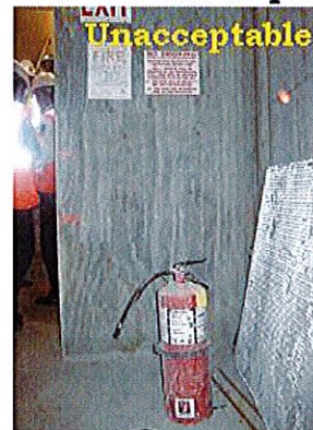
Improper floor placement of Fire Extinguisher.
